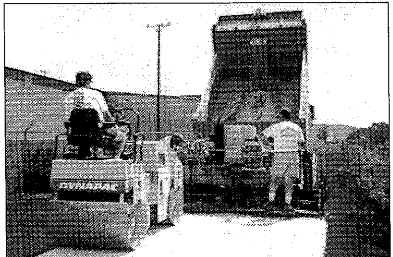
A paving crew works to make progress on the Five Star Trail section.
